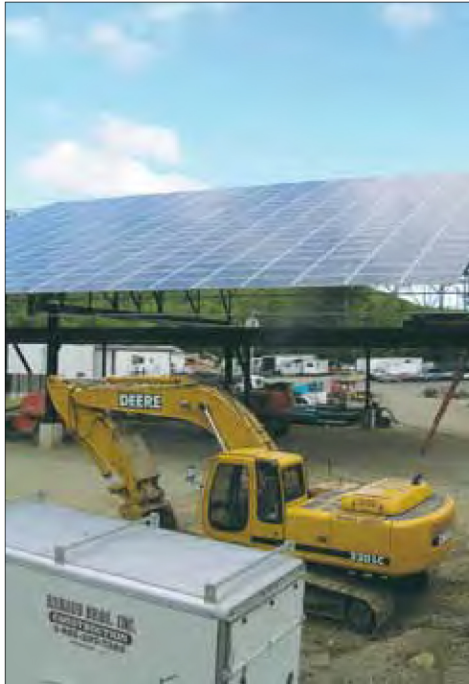
The dual purpose Commercial Car Port provides a new roof space with direct access to the sun for the solar project, as well as a place to park their commercial vehicles.
