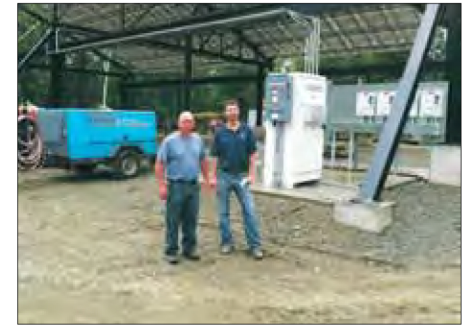
From left to right: Mike Renaud, Vice President and owner of Renaud Brothers, Inc. and Mike Whigham, lead designer with Integrated Solar are standing in front of the Solectria inverter and combiner boxes. Above them you can see the back of the array.
