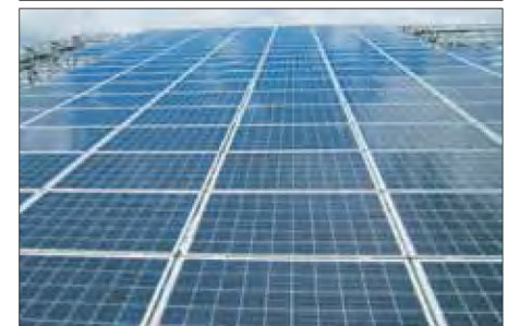
'Reaching for the Sky' at Renaud Bros., with the 312 SolarWorld modules that complete the 74.88kW solar photovoltaic system.
